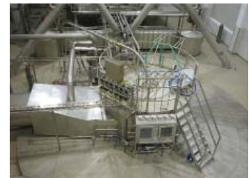
Bottom part of the CIP cleanable back house filter and conical part of the dryer (left)
