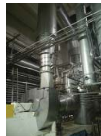
MVR Evaporator on a Whey Plant
