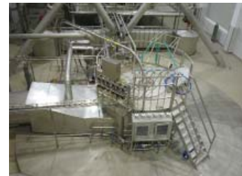
Top of Triple A Spray Dryer
