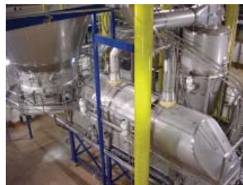
Triple A Dryer with integrated fluid bed and external fluid bed
